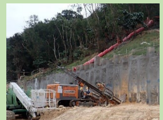
安裝挖掘與側向支撐系統上的錨杆 Installation of Tieback of Excavation and Lateral Support System
