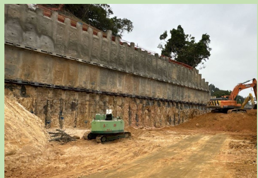
挖掘及安裝挖掘與側向支撐系統 Excavation and Installation of Excavation and Lateral Support System
